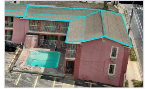
Fig. 3 Main building, east wing. Lifted caps along the hip ridges.
